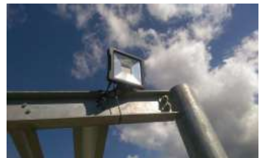
Brand new LED flood lights
