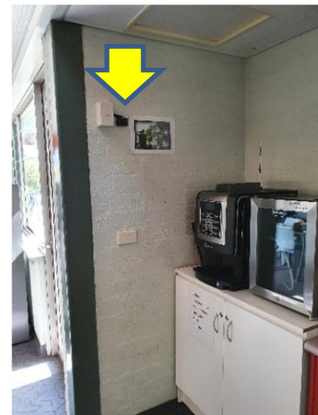
The Dining Room siren is located near the coffee machine
